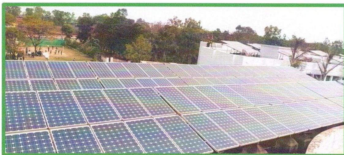
Figure 3: Rooftop Solar Panel
